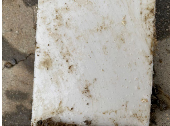
Figure 98: Closeup of formulation 3 surface showing blistering and air bubbles in coating.
