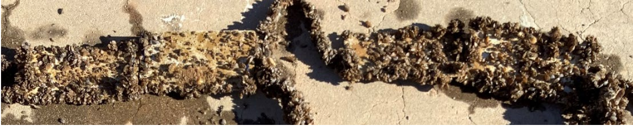
Figure 70: NDSU 4 (left two panels) and NDSU 5 (right two panels) in static testing conditions January 2022 inspection.
