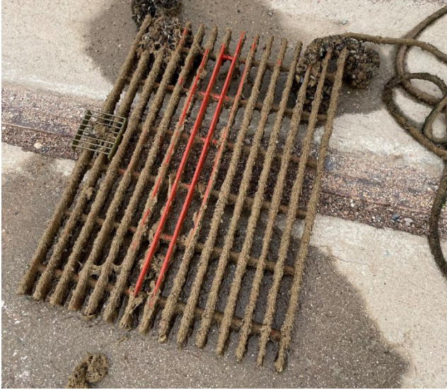
Figure 6: Jotun Repulse during July 2022 inspection with accumulation of colonial hydroid on surface of grate.
