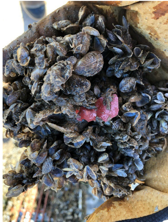
Figure 14: Piece of topcoat of Jotun Sealion Resilient that has flaked off.
