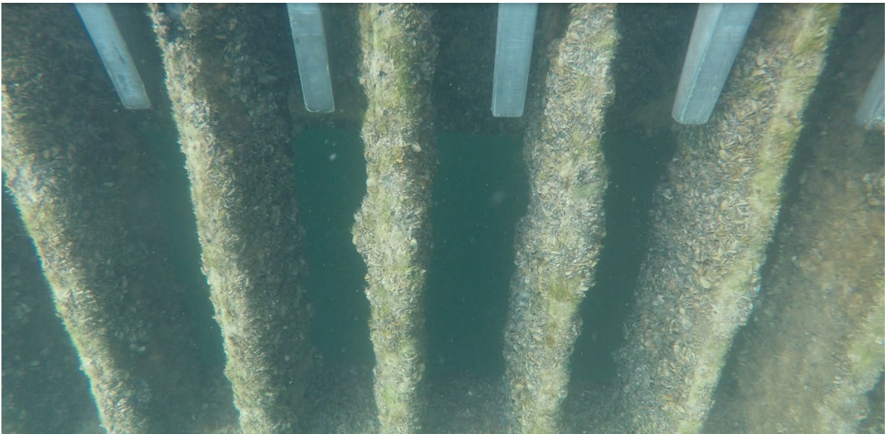
Figure 110: Section of trashrack not coated with FRC that is 100% fouled with mussels.
