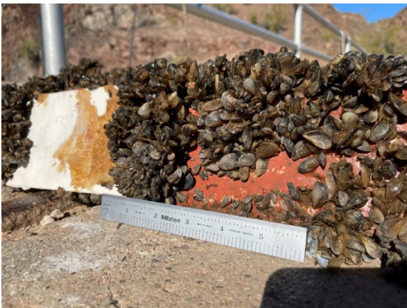
Figure 56: NDSU 8 (left) NDSU 9 (right) test panels in dynamic conditions. NDSU 8 remained free of fouling since the January inspection. NDSU 9 was fouled but easily cleaned. NDSU 9 also had some damage to the topcoat.
