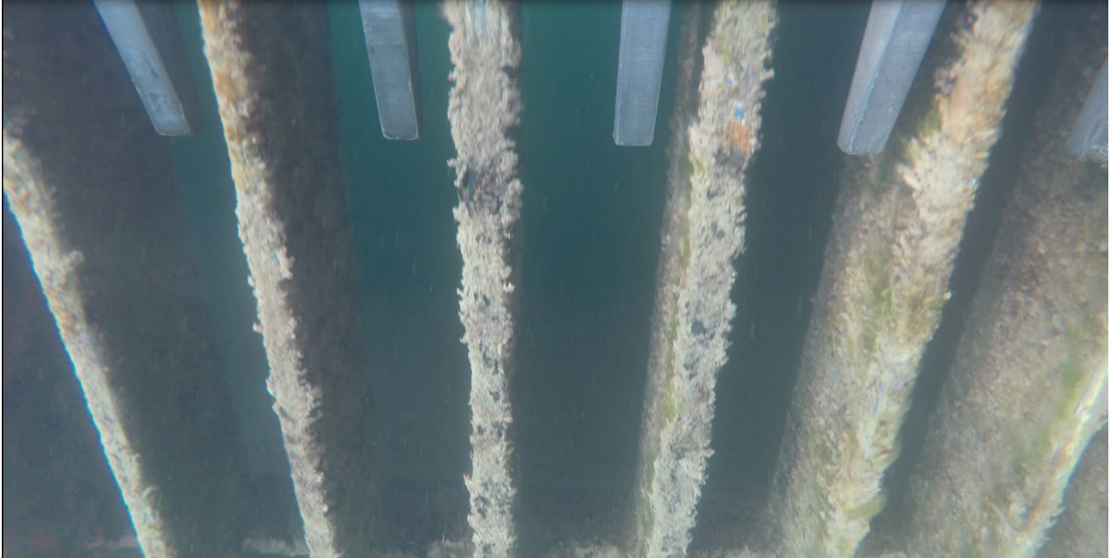
Figure 109: Seaspeed V5 which has become covered in algae but still prevents mussel attachment. The coating is damaged with missing spots of coating and corrosion present.
