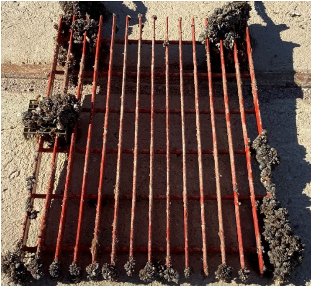
Figure 4: Jotun Sealion Repulse flowing water test grate during January 2022 inspection. No fouling except for areas of damaged coating.
