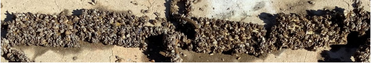
Figure 71: NDSU 6 (left two panels) and NDSU 7 (right two panels) in static conditions January 2022 inspection.
