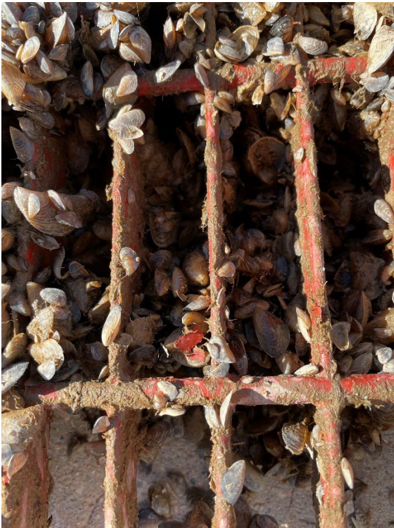
Figure 13: Damage to Jotun Sealion Resilient with topcoat flaking off.
