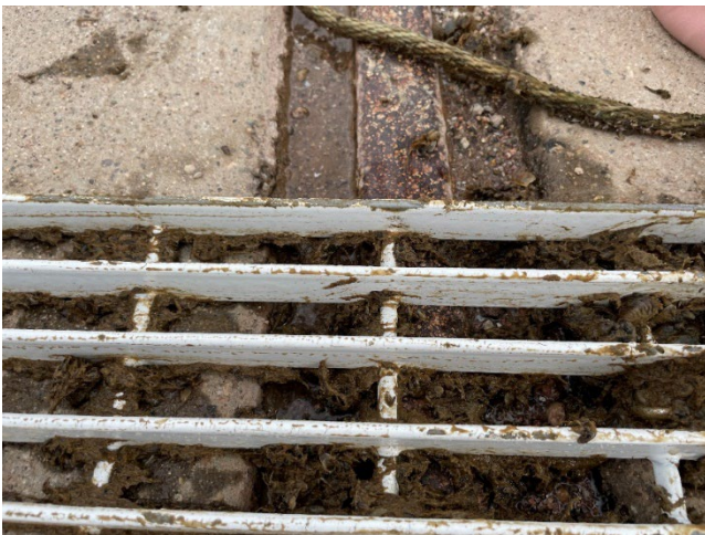
Figure 30: Damage and missing coating observed on edge of Sigmaglide 890 grate during July 2022 inspection.
