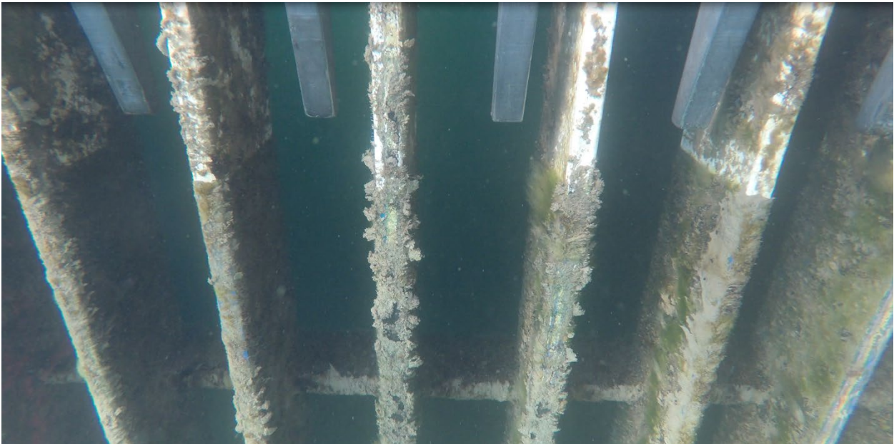
Figure 108: Sher-release and Seaspeed V5 interface. The bearing bars for the Seaspeed have abrasion damage and the coating has allowed for more accumulation of algae.
