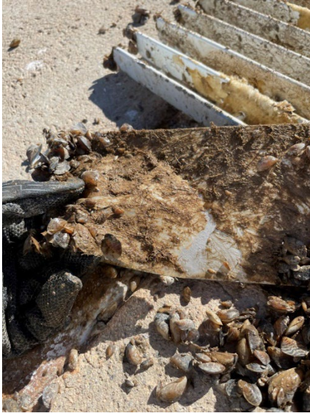
Figure 61: NDSU 3 panel where large portion of topcoat has delaminated in one piece.
