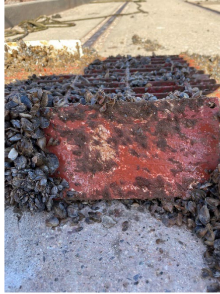
Figure 59: Close up of damage on NDSU 9 dynamic panel after cleaning during January 2022 inspection.
