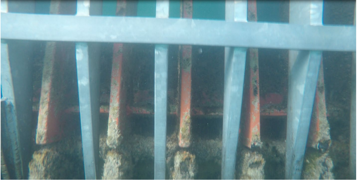
Figure 105: Bottom section of trashrack coated with Sigmaglide 890. Some missing coating at the bottom of the grate likely damaged by the rake system.
